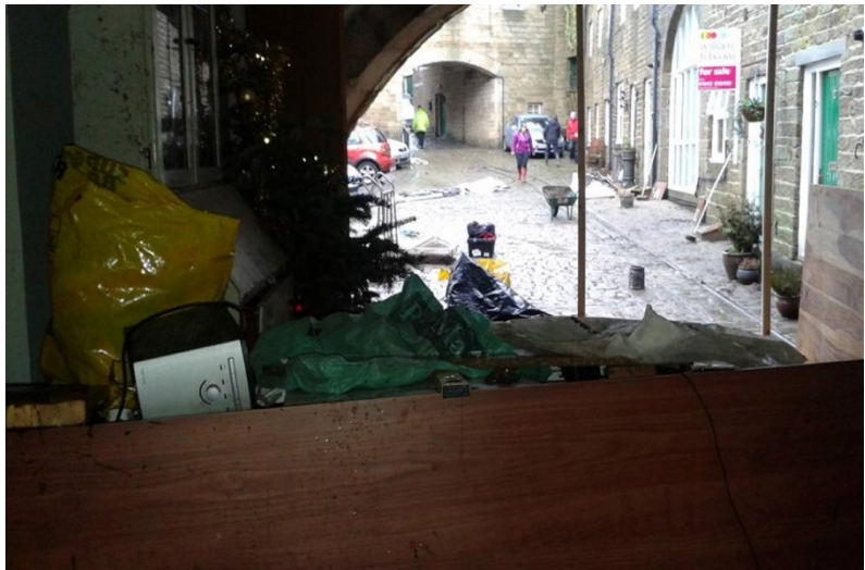
Flood Water destroys arch window in 2015 event.
