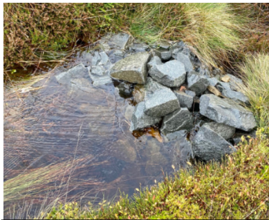
Leaky Dam Structure
