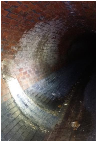
Outfall from Holiday Inn to Eastbrook with clear signs of pollution
